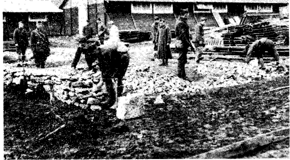
Engineers lay the foundation for a field hospital building at Méné-la-Tour (Meurthe-et-Moselle), France.
